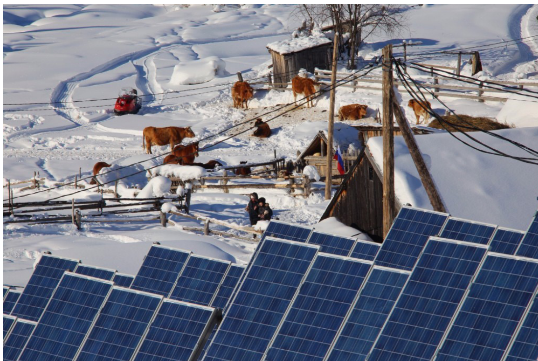
Fig. 5. Solar power plant. Yunkur village, Verkhoyansky district, Republic of Sakha (Yakutia) 5 .
